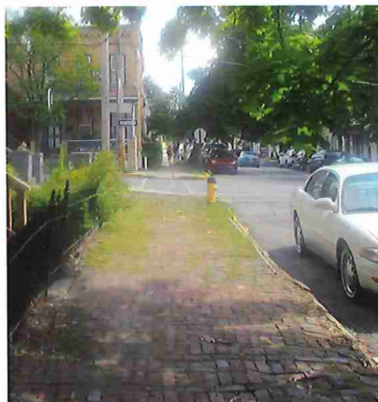
Brick Sidewalks like this along Mulberry Street give character to the neighborhood; however, they require additional maintenance to keep the surface condition even and safe.
